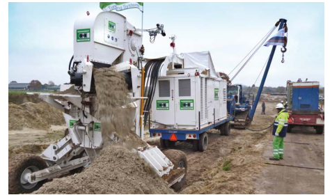
Surface vehicle with power unit compartment.
