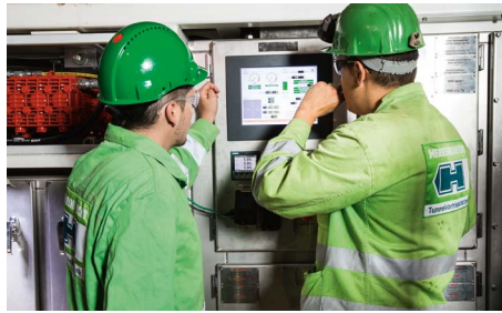
Power pack with PLC control and data recording system.
