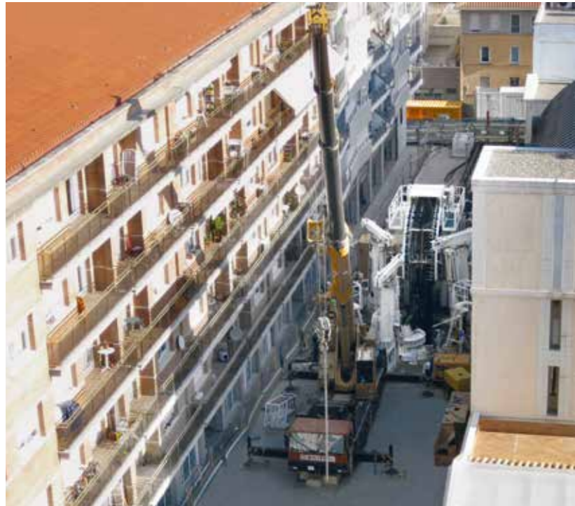
The flexible arrangement of the individual components makes it possible to lower shafts even in narrow streets that are only a few meters wide.
