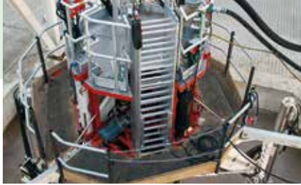
Control platform with access ladder.
