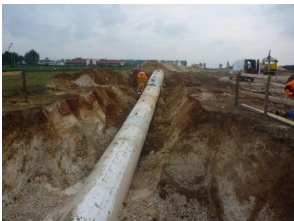
The pipeline precisely reached its target point at the opposite river side after more than 1,000 meters of tunnelling.
