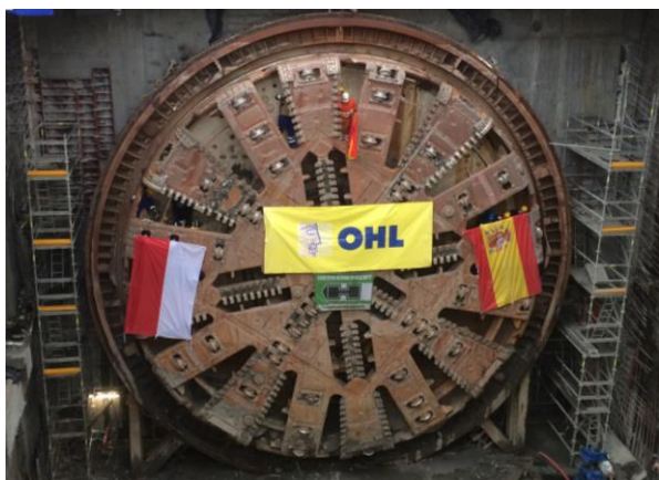
Photo 2: The breakthrough of the first tube took place in November 2013. The final breakthrough was achieved in June 2014.
