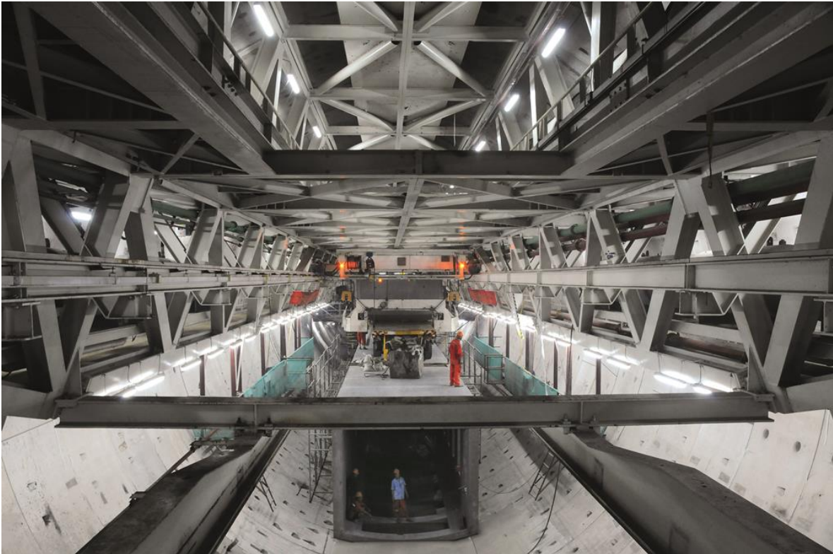
Picture 2: Rear view of the world's largest Mixshield TBM S-593 under Qiantang River.
