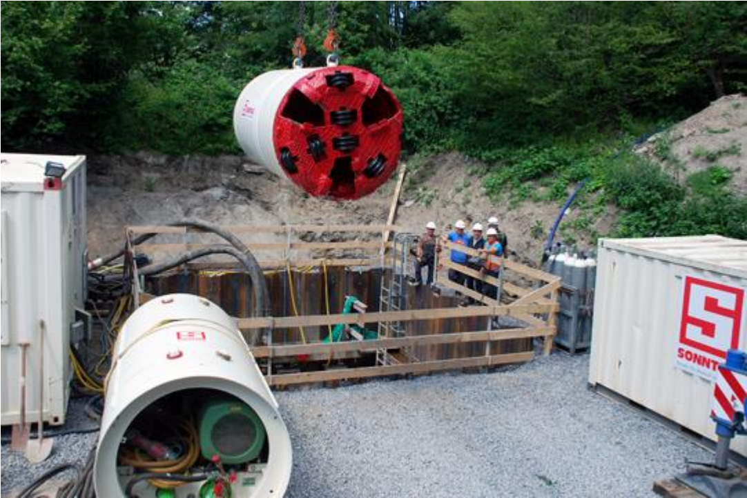
The AVN machine with a bore diameter of 1,505 millimeters finished a total of 6 drives in Karlsruhe.
