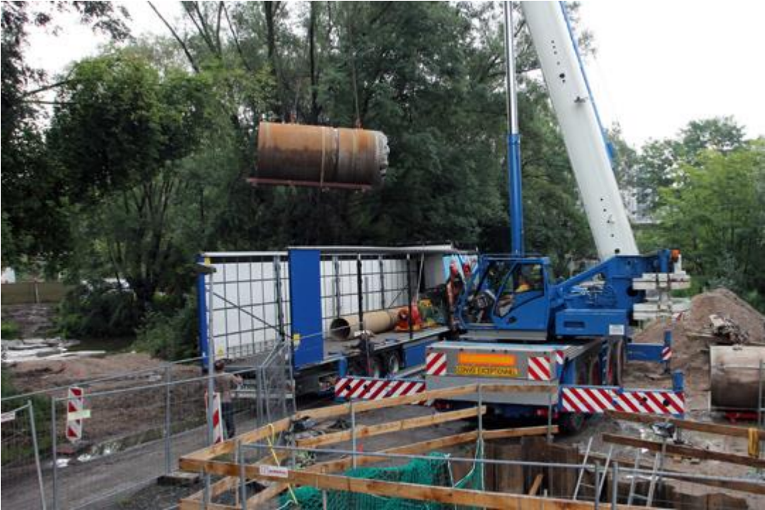
After breakthrough and completion of the 110-meter-long alignment, the AVN1200 is transported from the target shaft to the next construction site. In the distance on the left in the picture, the successfully crossed "Alb" creek.
