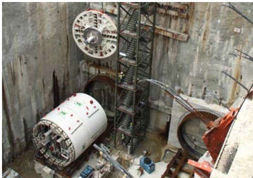
Photo 2: The Herrenknecht TBM S-774 during assembly in the Cochrane launch shaft. From here it excavated a total of 4.4 km of tunnel right through the center of Kuala Lumpur. Half of that through karstified limestone as a Mixshield with variable adaptation of the suspension density. For the second part through the softer mixed geology of the Kenny Hill Formation the machine was switched to EPB mode.
