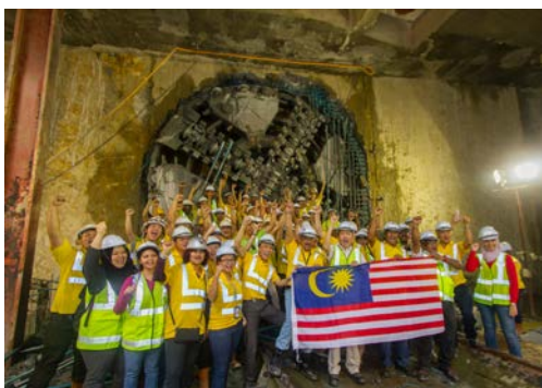
Photo 4: An innovation celebrates its breakthrough: with the arrival of the Herrenknecht Variable Density S-774 on April 11, 2015 all tunnelling work for Kuala Lumpur's first metro has been completed. At the same time an innovative technology has created facts and demonstrated new possibilities in mechanized tunnelling.
