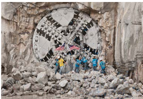
Photo 3: Breakthrough of the Herrenknecht TBM S-776 into the Passar Rakyat station on January 9, 2014. The sister machine S-774 continued through the station and excavated a second and third section. On their way the machines crossed under the SMART tunnel built by two Herrenknecht Mixshields nearly ten years previously. The experience gained at that time was incorporated into the development of the Variable Density TBM.
