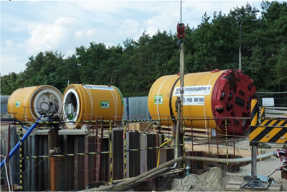
Ready to go: the Herrenknecht AVND2400AB for the underground connection of a new wastewater treatment plant in Warsaw, Poland.
