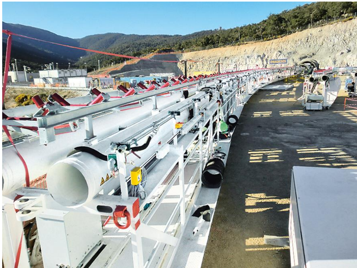
The back-up systems of the two Double Shield TBMs are designed for high tunnelling performances, allowing the storage of the segments and other material for two ring building sequences.
