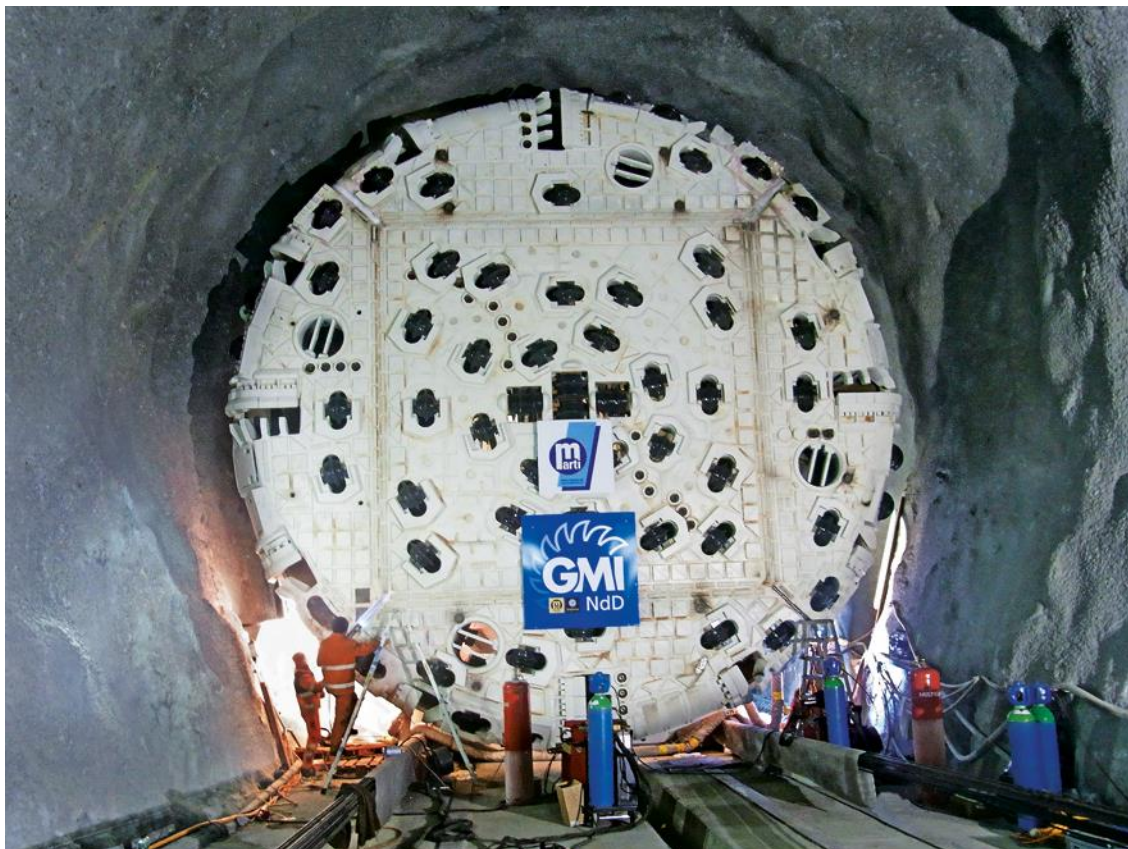
The Gripper TBM S-522 (Ø 9,450mm) is in the launch position to excavate the over five kilometer long access tunnel.
