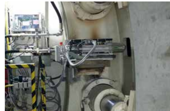
The impact hammer generates seismic waves into the tunnel rock wall after each stroke or ring.
